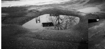
Frost heaving problems
